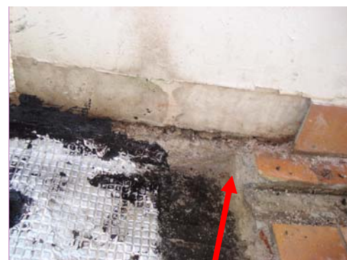
Terrasse MOMBELLI - Absence de joint
